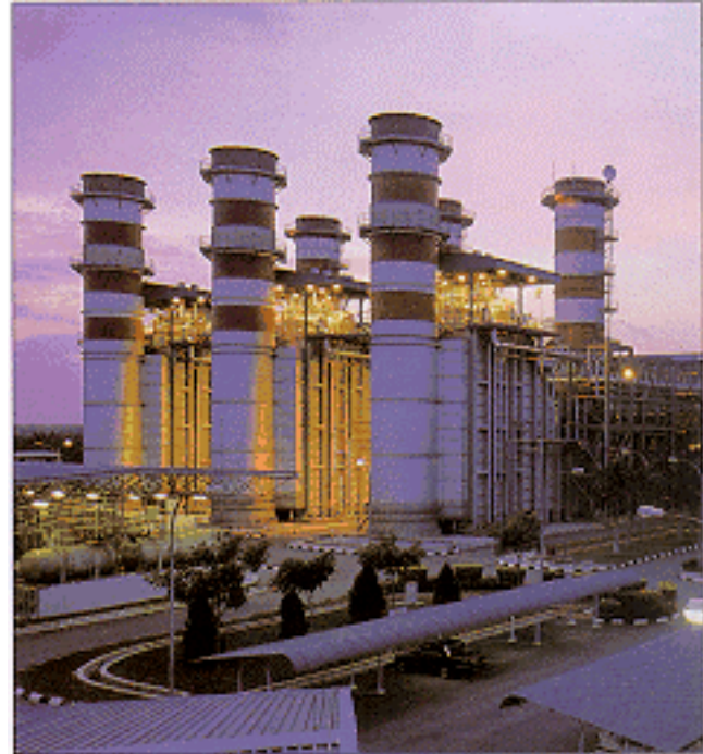
Power plant at Kuala Langat, Selangor
