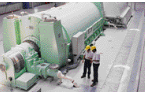
Steam turbine generator
