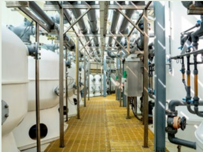
Seawater storage tanks
